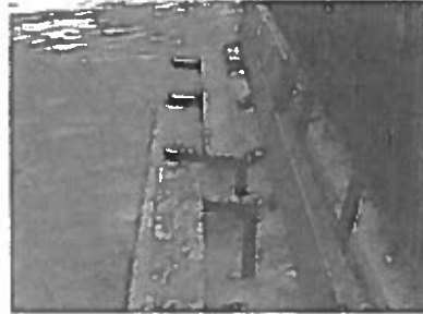
Benches missing slats
