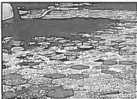
Paved surface with deterioration of hex blocks
