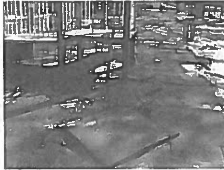
Safety surface damaged in a critical area of the playground
