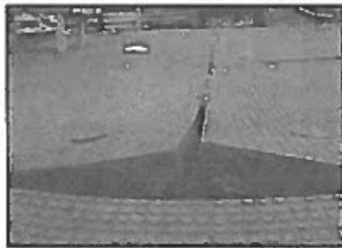
Safety surface uplifted causing safety hazard
