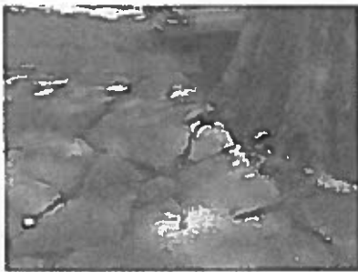
Severe trip hazard on sidewalk
