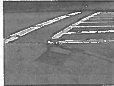
Sidewalk trip hazard
